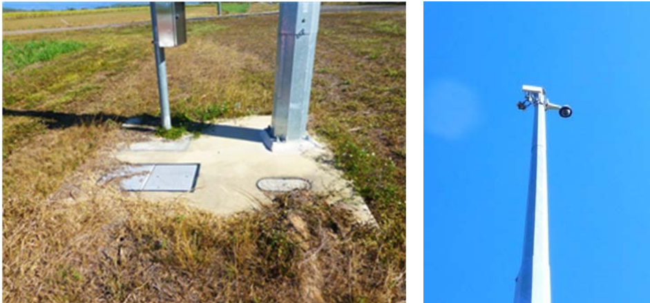
Figure 9 - TMR Camera Pole (at Chainage 109,900m)
