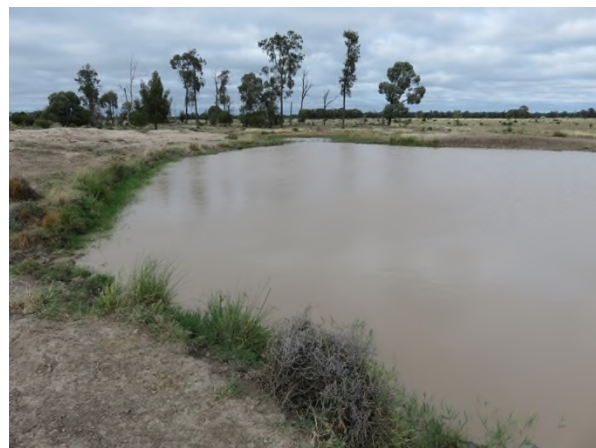
Plate 10 – Disturbed gilgai from earthworks
