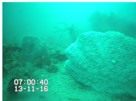
Plate 3-4 Observations of the marine environment at the base of the ship loader piles and growth on the piles
