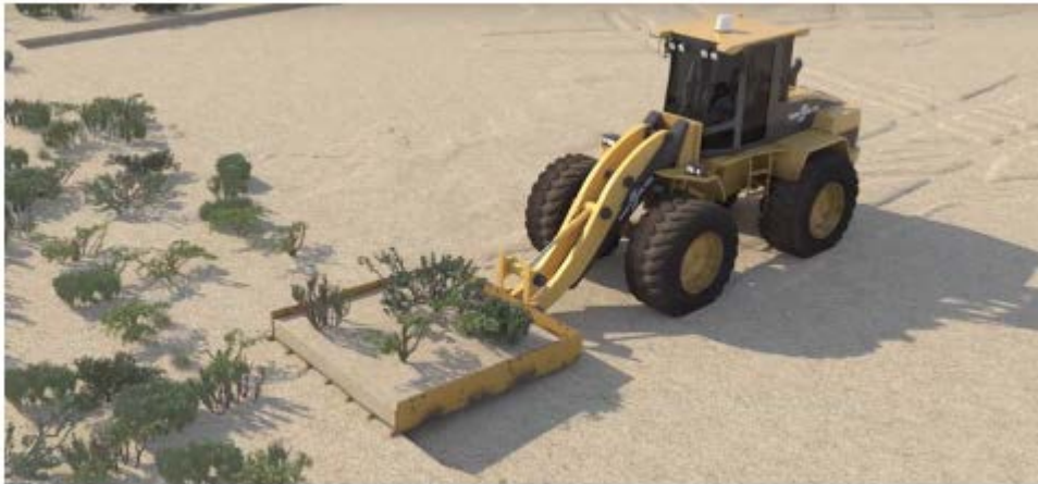
Figure 2: Sod removal of the VDT process using a modified front end loader
