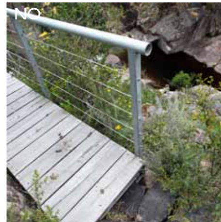
IMG1584 - Lack of end cap unappealing
