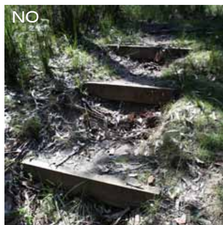
IMG 1974 - Timber steps with erosion
