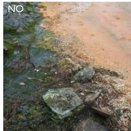
IMG 5836 - Water bypassing culvert
