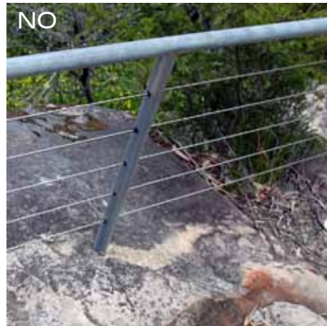
IMG1604 - Leaching from galvanised handrail
