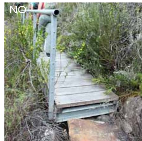
IMG 1582 - Poor edge interface with Trail
