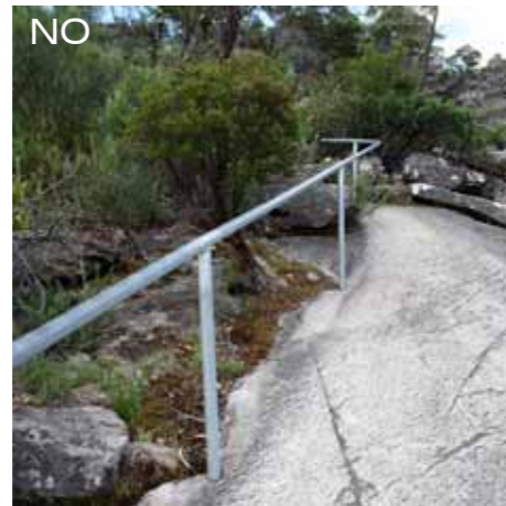
IMG1697 - Unnecessary handrail
