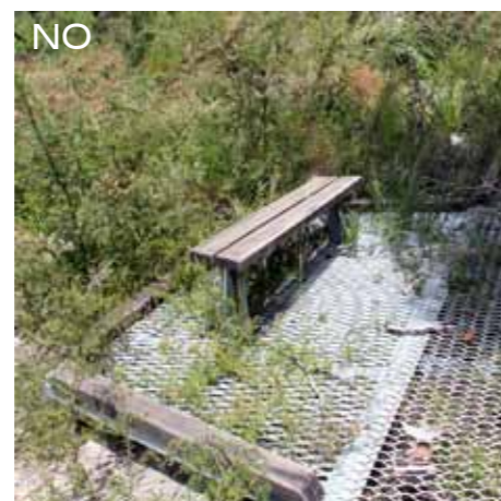
IMG 1667 - Seat too constructed / out of place
