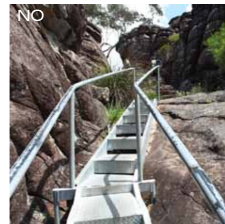
IMG 1650 - Excessive use of steel
