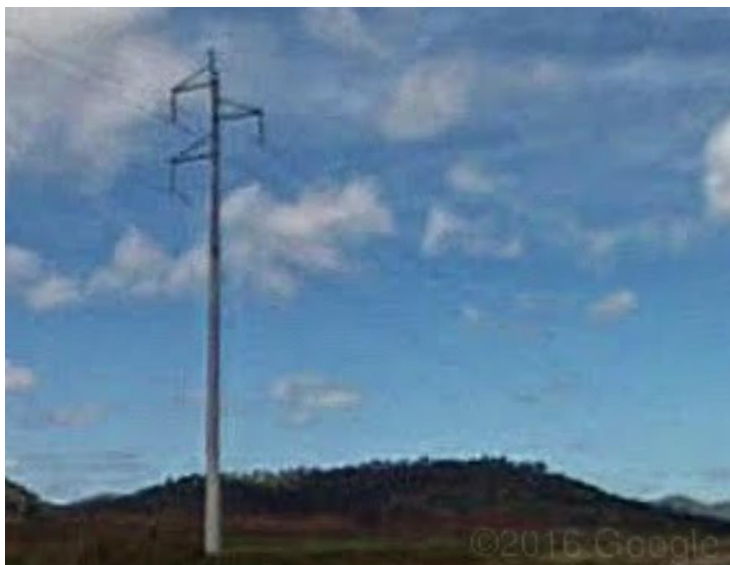
FIGURE A-8: ERGON 132kV POWERLINE SOUTH OF LAKELAND
