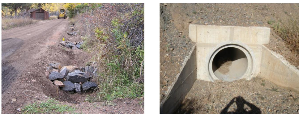
FIGURE A-3: IMAGES OF TYPICAL ACCESS ROAD DRAINAGE. LEFT: ROAD SIDE DITCH WITH SIMPLE DETENTION FACILITIES. RIGHT: CONCRETE CULVERT WITH SUPPORT STRUCTURE
